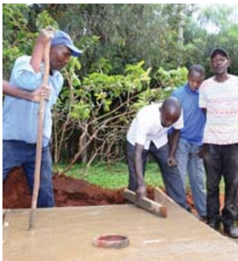
WASHplus teaches its trainees to create a sloping concrete slab to facilitate clean up.
