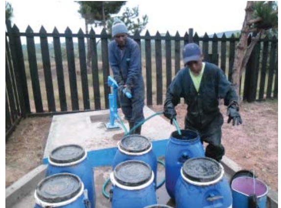
Workers from the local service provider, Aina, disinfect equipment used to extract and transport sludge to the burial site. The availability of water at the burial site is critical to ensure hygienic conditions.
